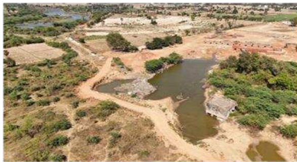
Breach portion in Right Side Flood Bank at Somanjeri during flood
