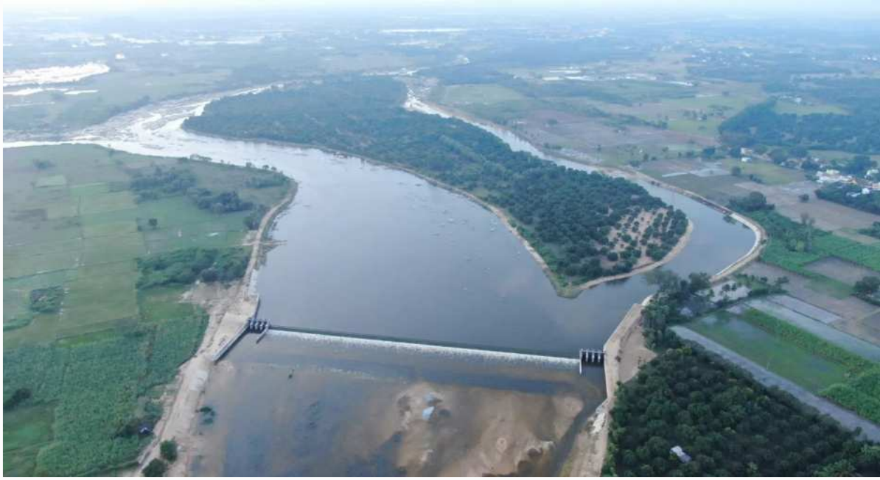
Construction of a Check Dam across the Cooum River near Soranjeri Village in Poonamallee Taluk of Thiruvallur District.
