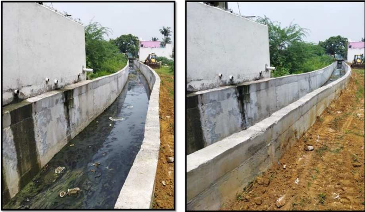
Construction of Storm water drain at MGR Nagar towards Kavarapalayam to Villinjiyambakkam lake in Ward no 22
