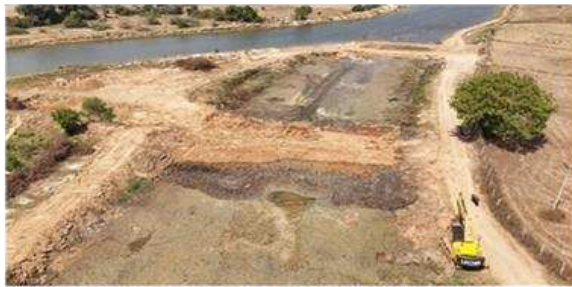
Breach portion in Left Side Flood Bank at Thattamanji during flood
