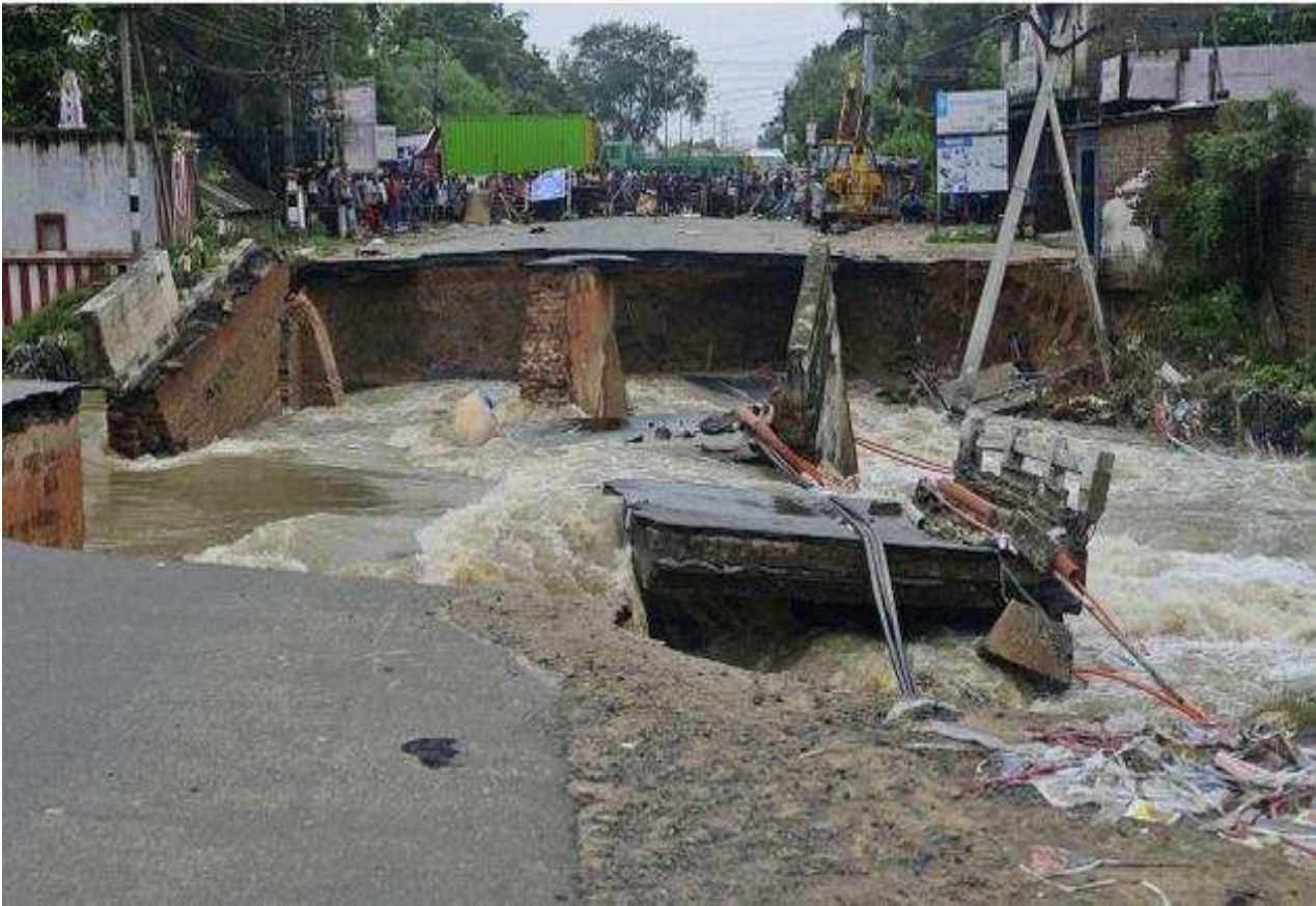
Damaged bridge on the Avadi-Poonamallee High Road
