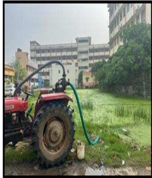
BAILING OUT WATER USING DIESEL ENGINE AT SARASWATHI NAGAR, ZONE -3 (WARD NO:42)
