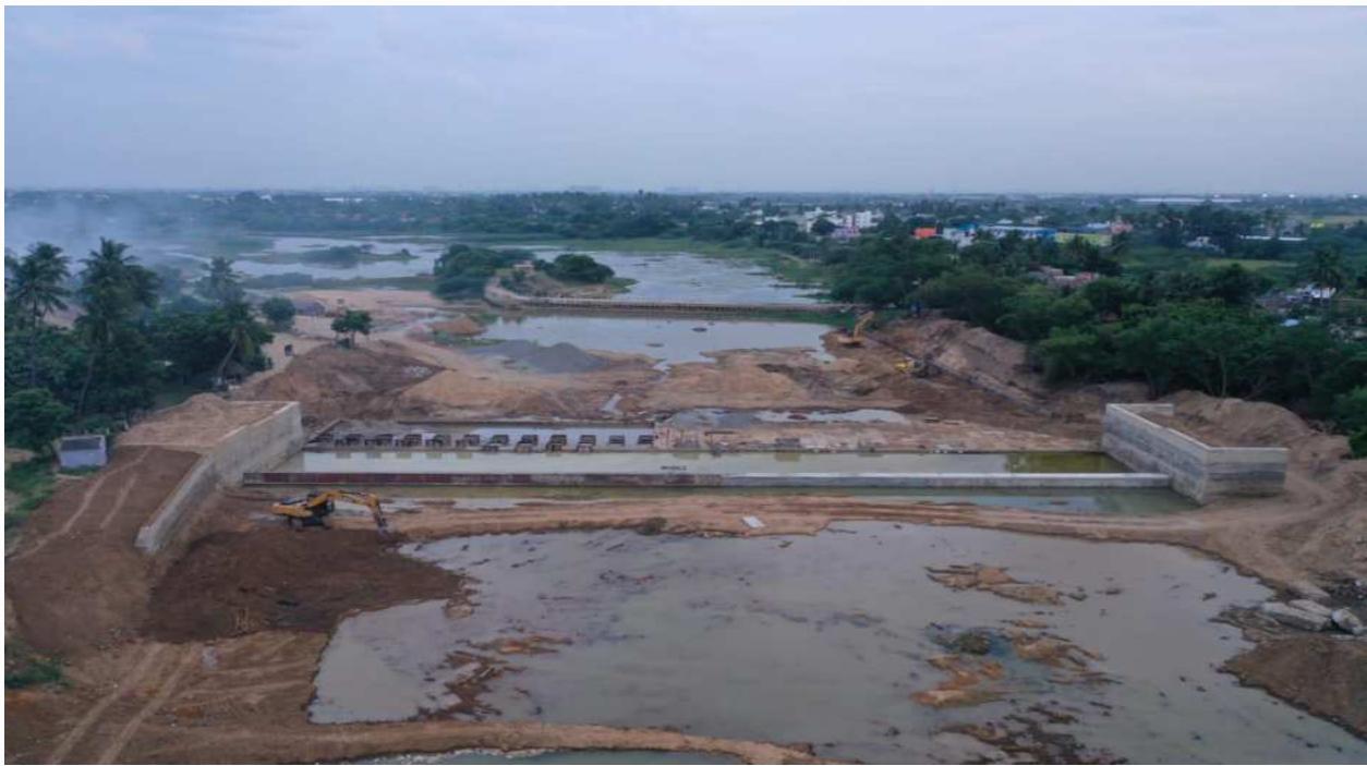
Construction of Check Dam Across Cooum river Near Athigathur Village in Thiruvallur Taluk of Thiruvallur District.
