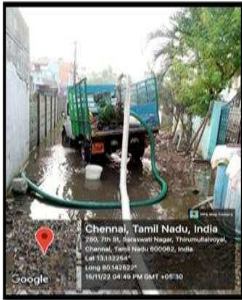
BAILING OUT WATER USING DIESEL ENGINE SARASWATHI NAGAR 7 TH STREET, ZONE -2 (WARD NO:29)
