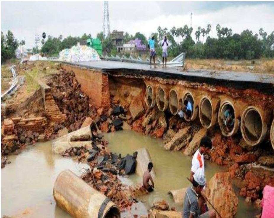
Periyapalayam – Tiruninravur – Jamin Korattur connecting bridge at Pudhuchatram in Tiruvallur district, (State Highway – 50A) damaged due to heavy rains.
