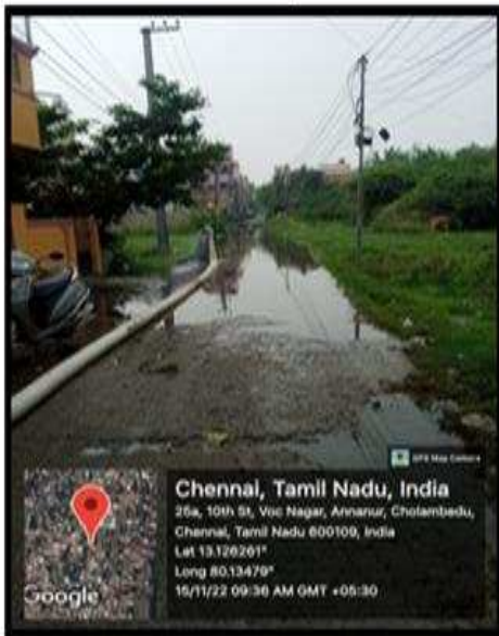
BAILING OUT WATER USING DIESEL ENGINE AT VOC NAGAR, ZONE -2 (WARD NO:27)
