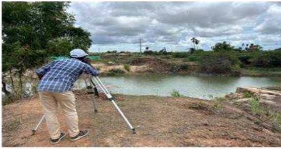
Breach portion in Right Side Flood Bank at Somanjeri during flood
