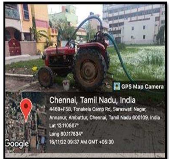
BAILING OUT WATER USING DIESEL ENGINE AT TONAKELA CAMP ROAD, ZONE -3 (WARD NO:42)
