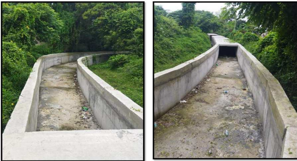
Construction of RCC Channel from Govindhathangal Lake to Villinjiyabakkam Lake in Ward no: 22
