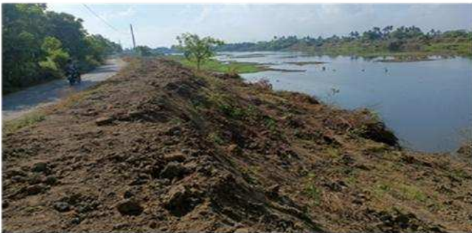
Slipped portion in Left Side Flood Bank at Nalur during flood
