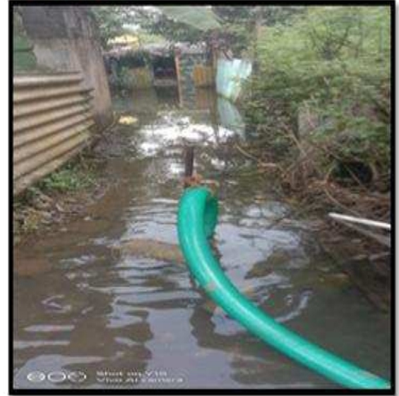
BAILING OUT WATER USING DIESEL ENGINE AT JOTHI NAGAR, ZONE -3 (WARD NO:33)
